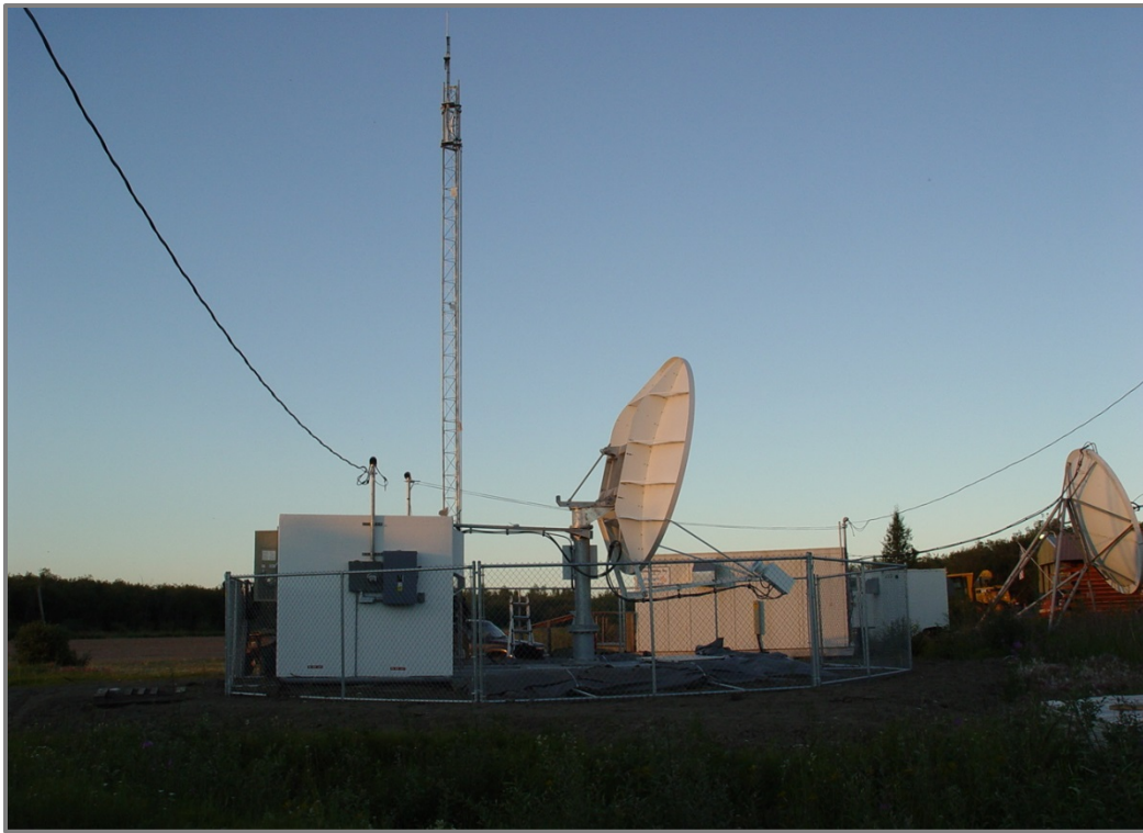
Photo 3: 3.6m Dish and Rohn 25G Antenna
