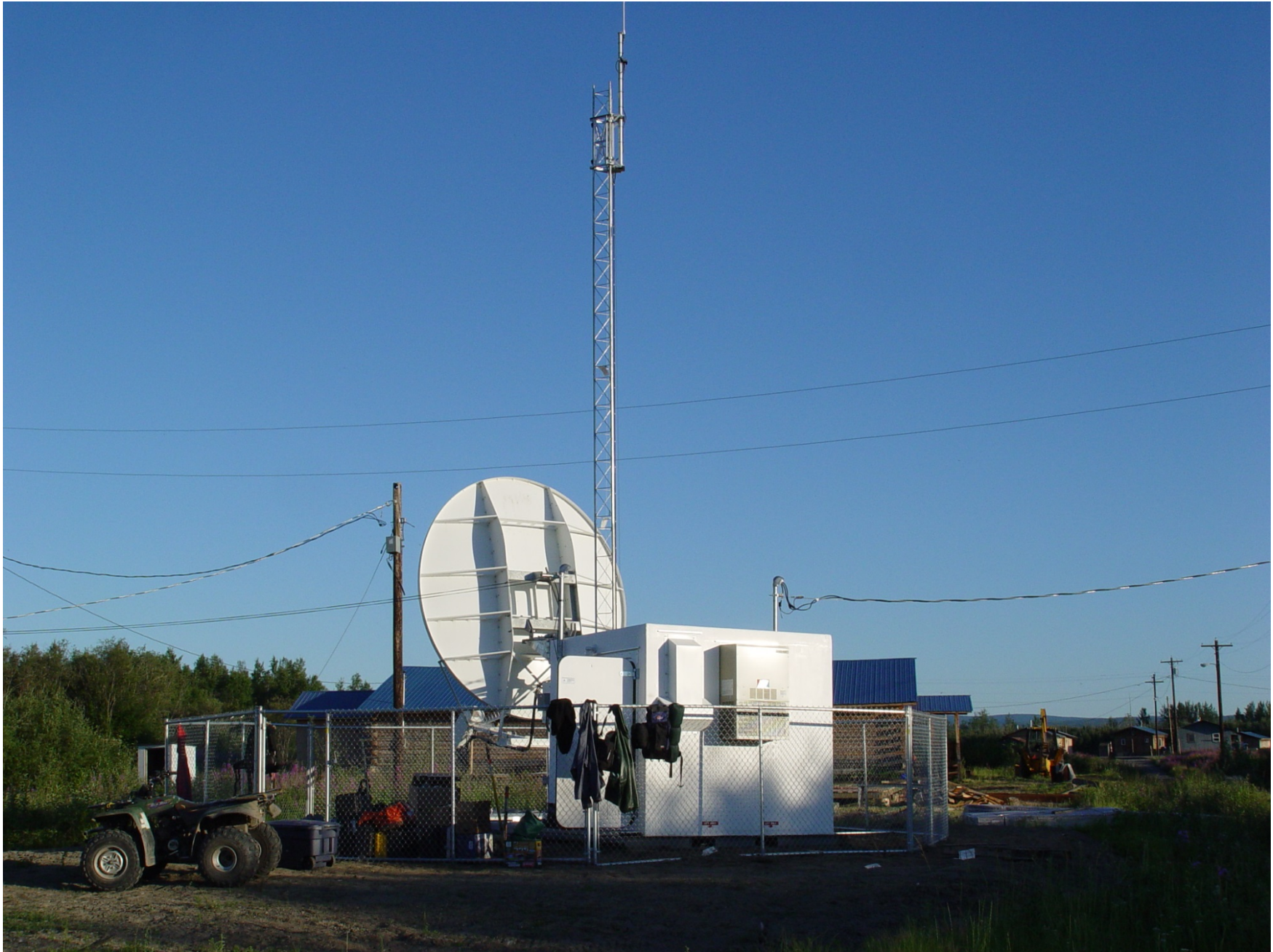
a. View of 3.6m dish. View to south.
