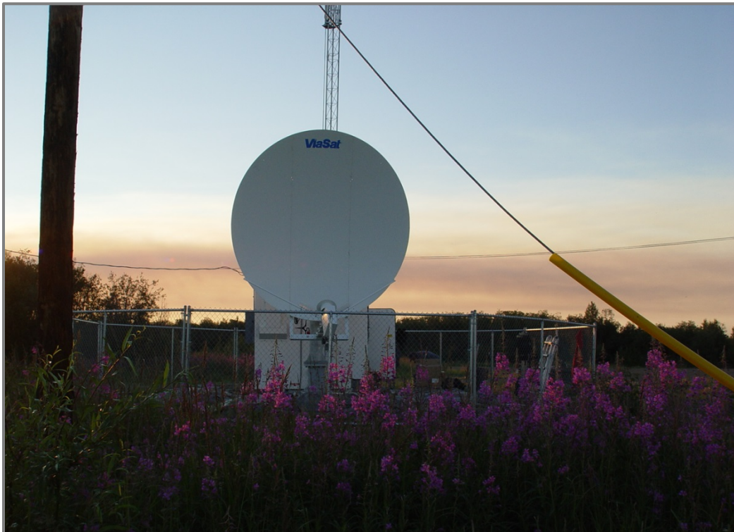
Photo 2: 3.6m Dish and Enclosure
