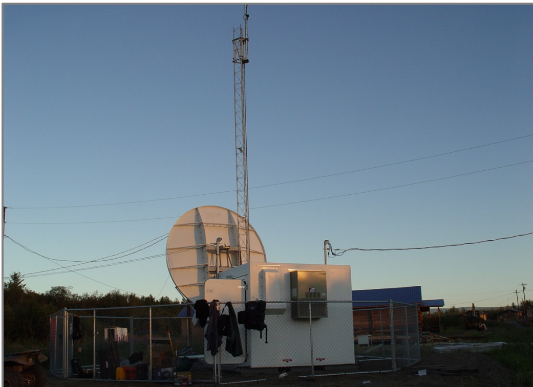
Photo 4: Stevens Village Telecommunications Facility
