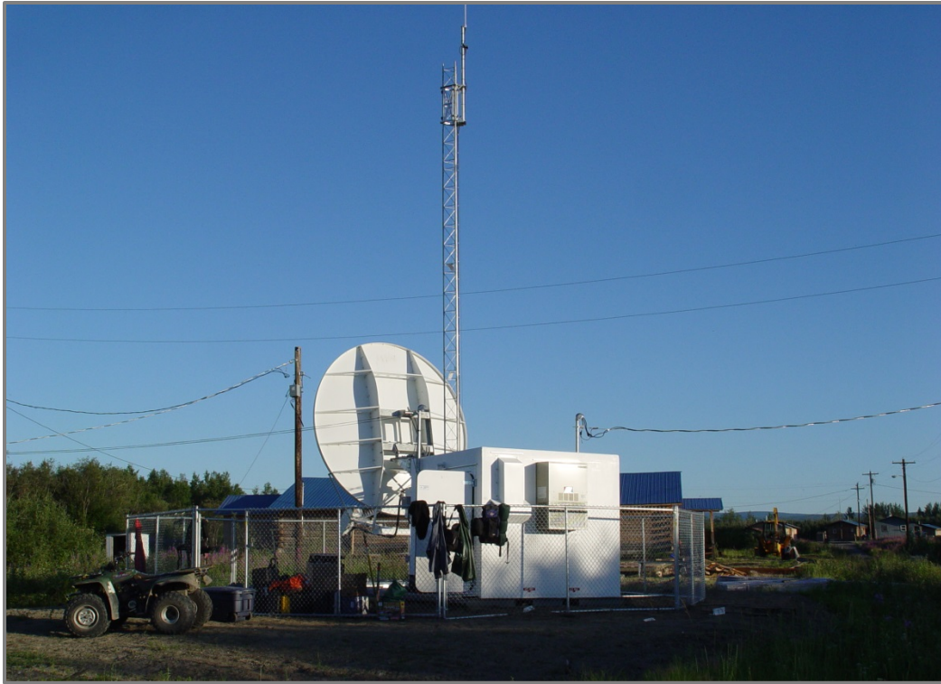
Photo 1: Stevens Village Telecommunications Facility
