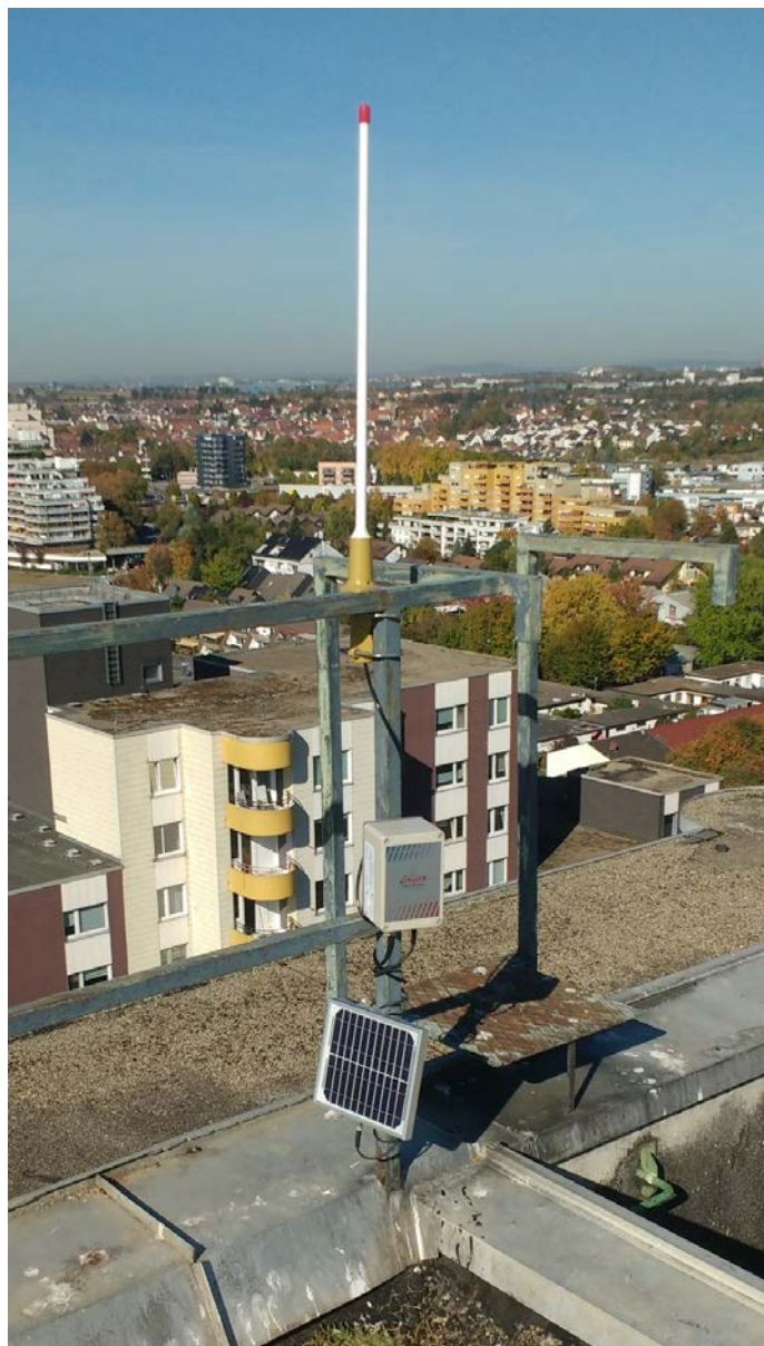
Sample installation with solar panel and rod antenna
