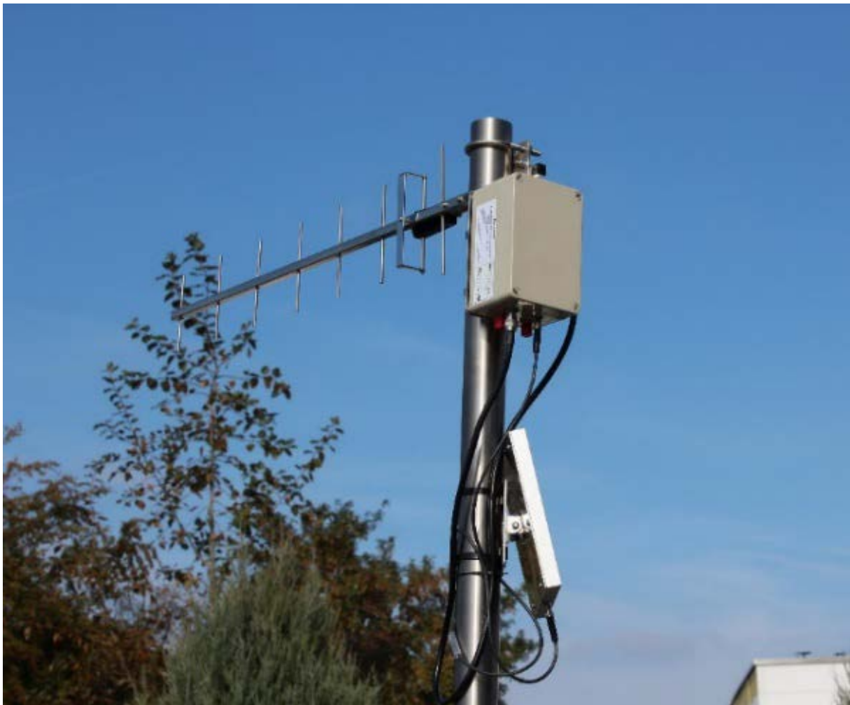
Sample installation with solar panel and Yagi
