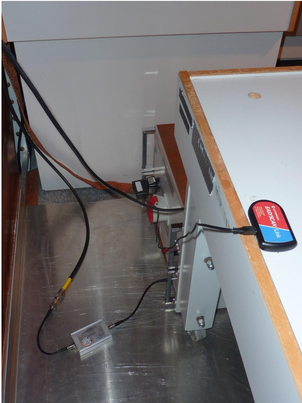
170032_f.JPG: EASYSCAN Link, test setup shielded chamber
