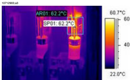
Figure 29.3 An infrared image of a fusebox where the maximum temperature is displayed
