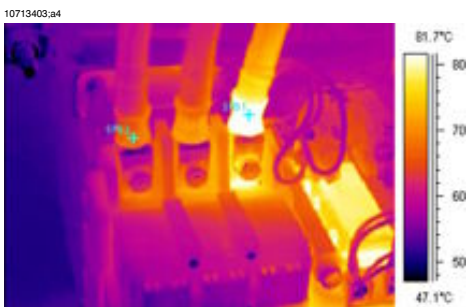
Figure 29.8 An infrared image of indoor electrical equipment (1).
