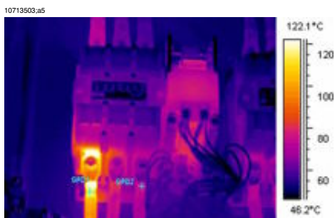
Figure 29.9 An infrared image of indoor electrical equipment (2).
