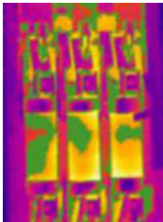
Figure 29.6 An isotherm in an infrared image of a fusebox
