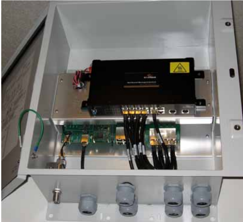
Figure 36 CMM4 (Cabinet with switch)
