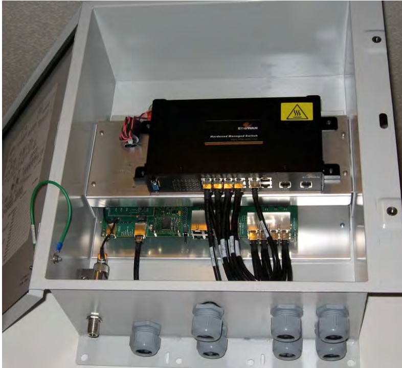
Figure 26 CMM4 (Cabinet with switch)
