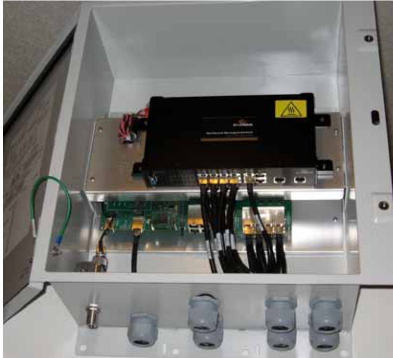
Figure 32 CMM4 (Cabinet with switch)
