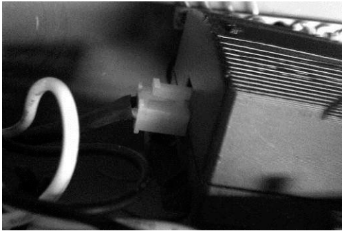
Power Cable attached to ePod
