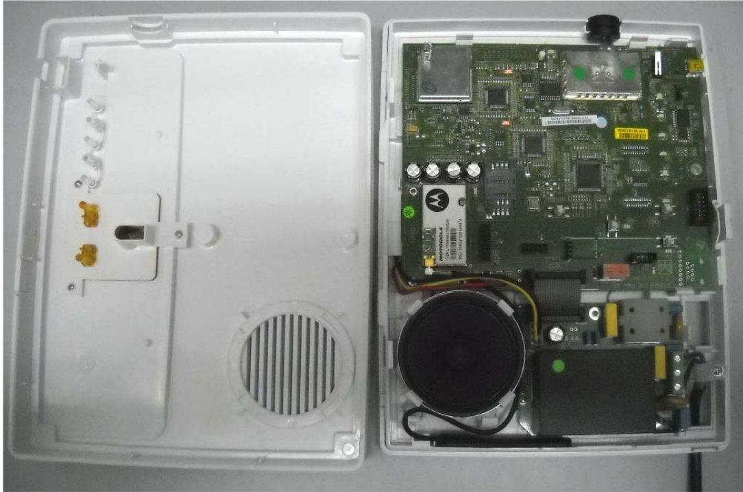
Photograph No.1 ES7000EG wireless control panel internal view
