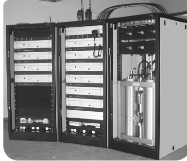
Figure 16 MX800 Setup in system rack
