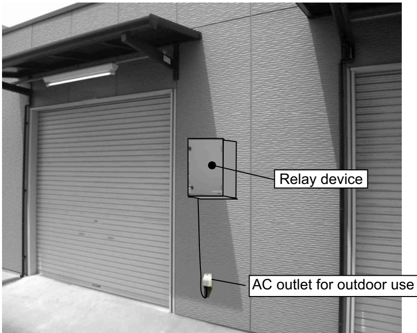
Relay device installed near the entrance to the cart barn
