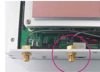
RF cable mounted at the front panel
