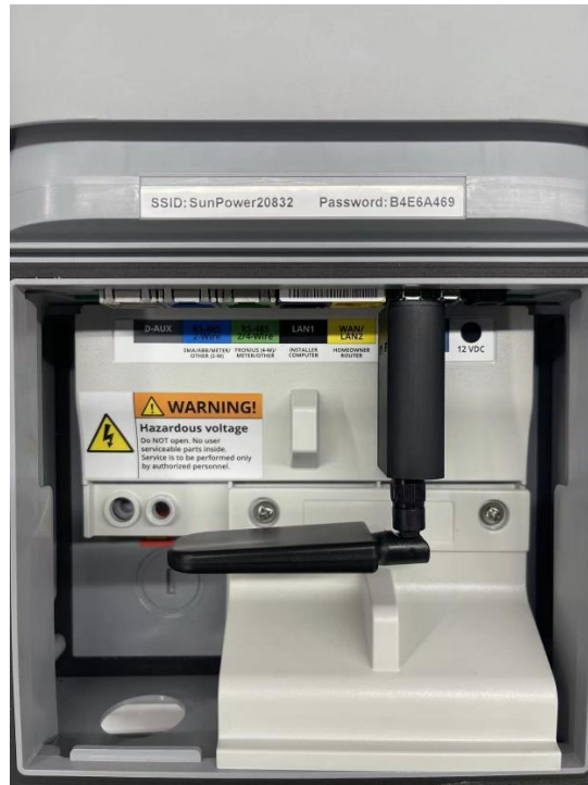
Photo 2.1: The communication module in the measurement meter
