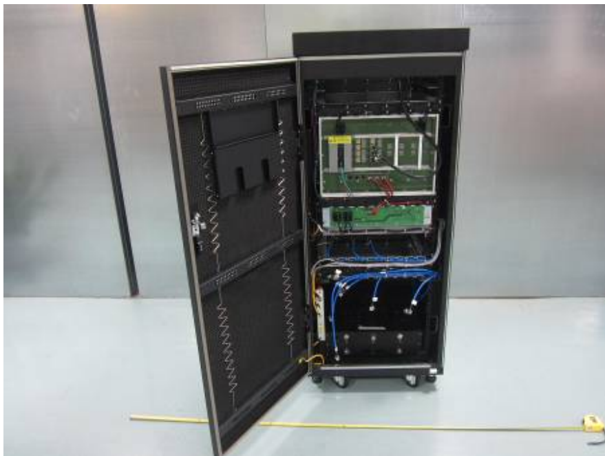
EUT – Rear Open View
