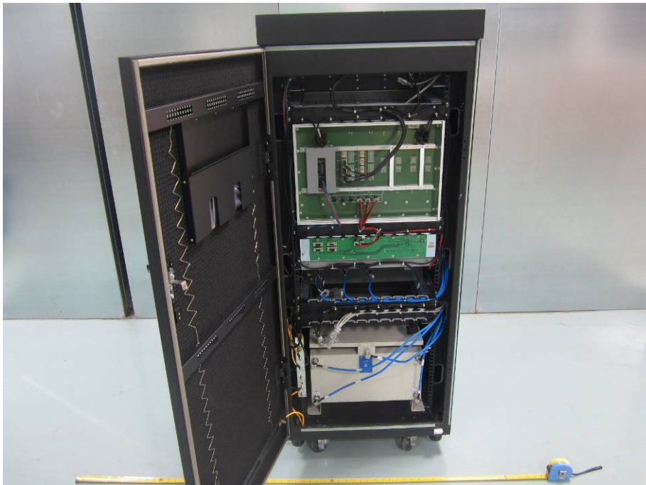
EUT – Rear Open View
