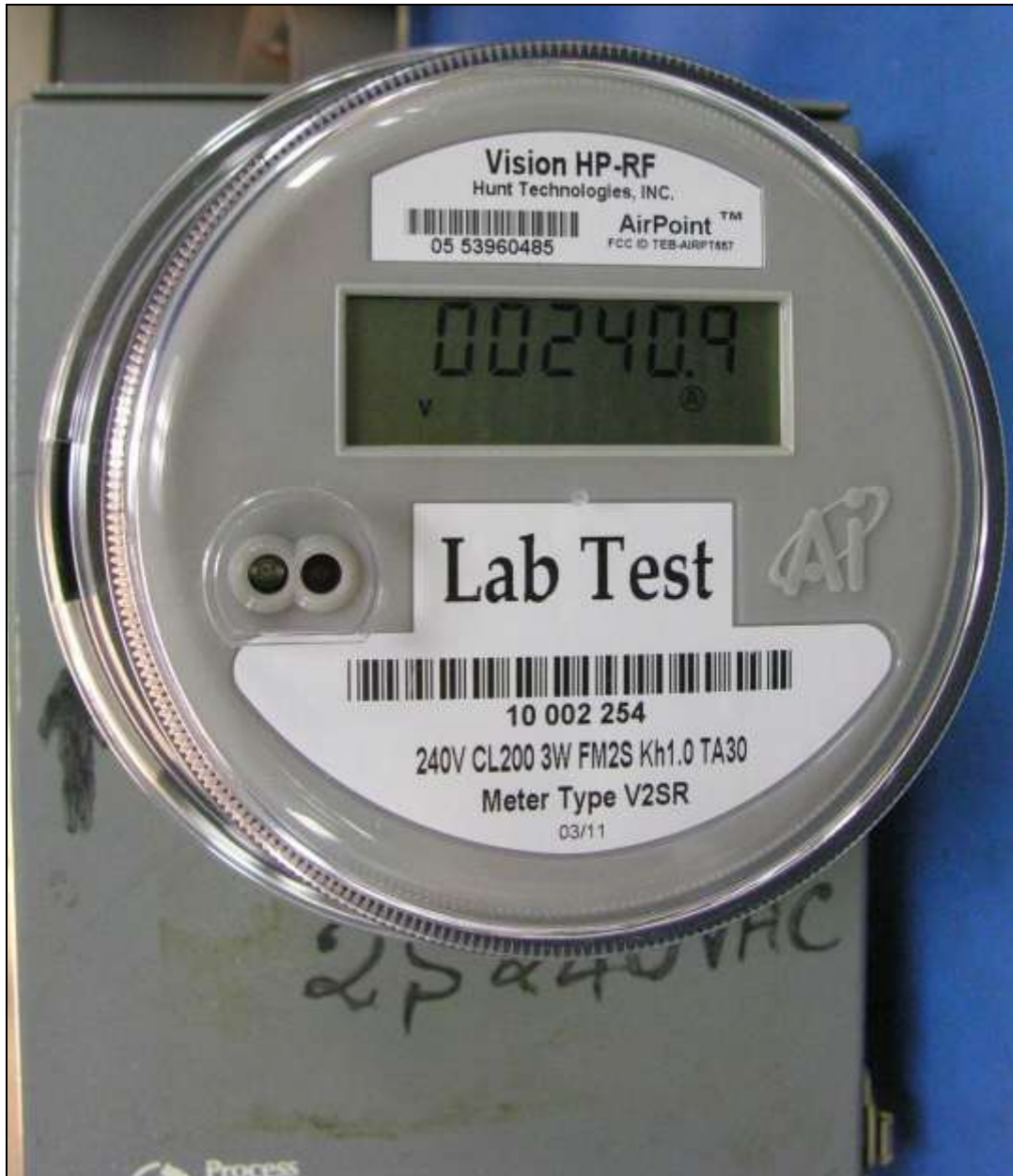
Photograph 1. Austin International, Inc. Two Phase Watt-hour Meter Model FM1S
