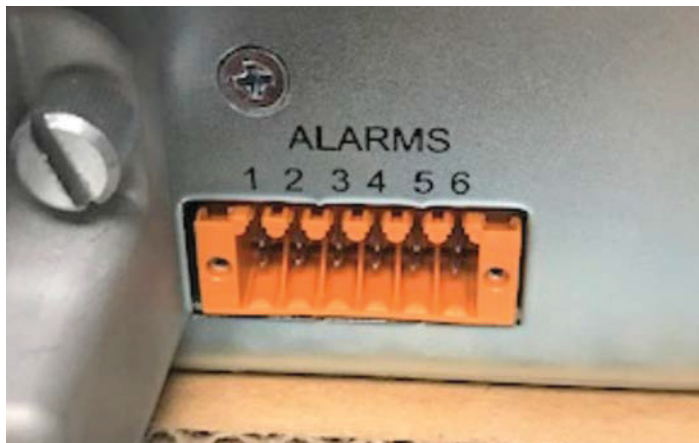
Alarm port on WCS back panel
