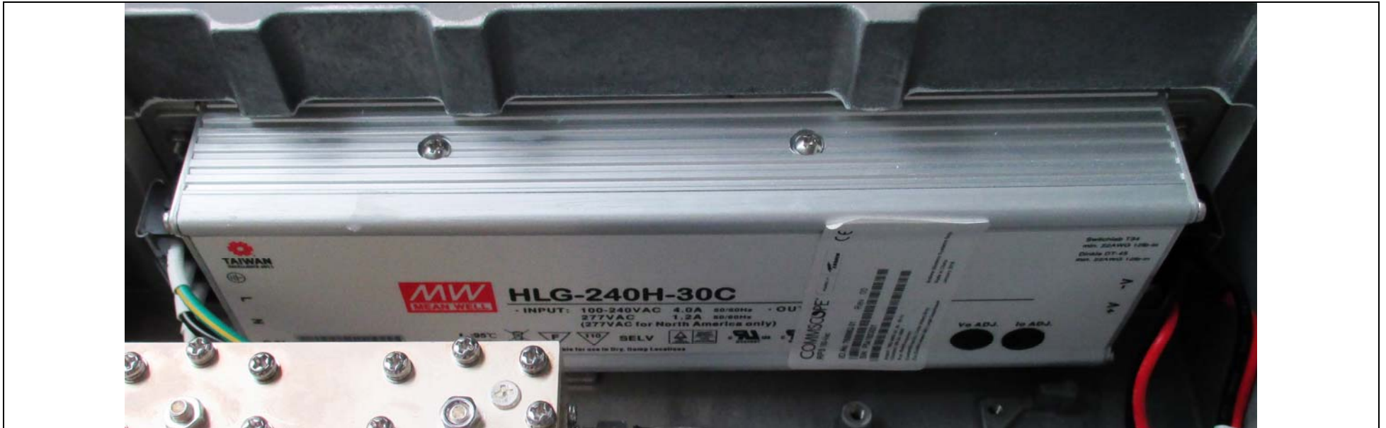
Power Supply Unit
