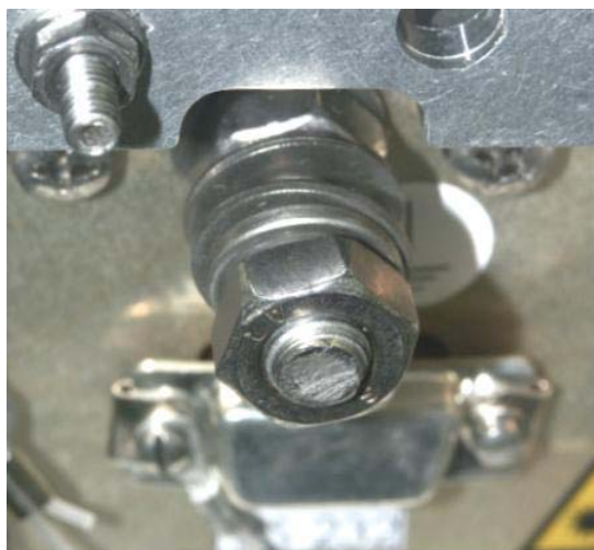
figure 3-7 Grounding bolt with loosened hex nut
