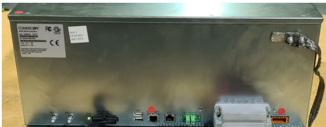
Photograph 6: Photograph of DUT's grounding
