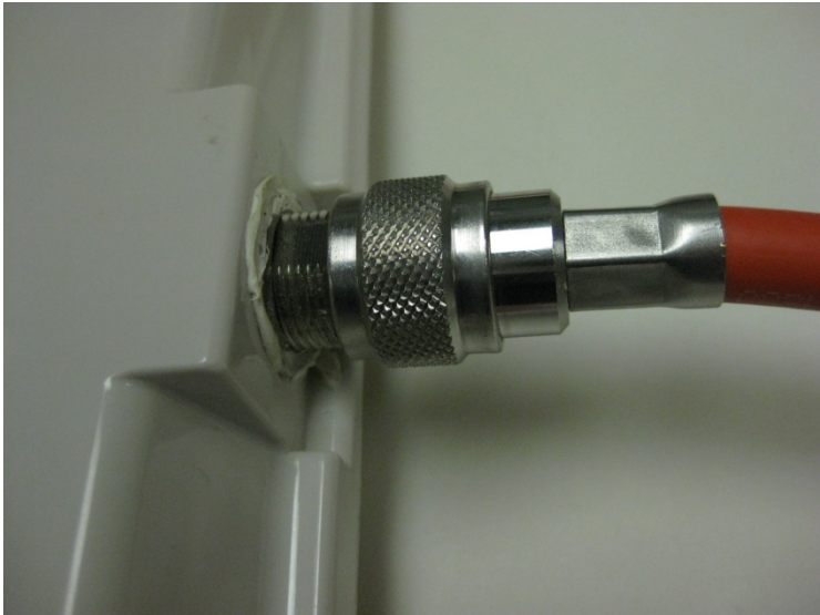
Antenna Connected to Cable
