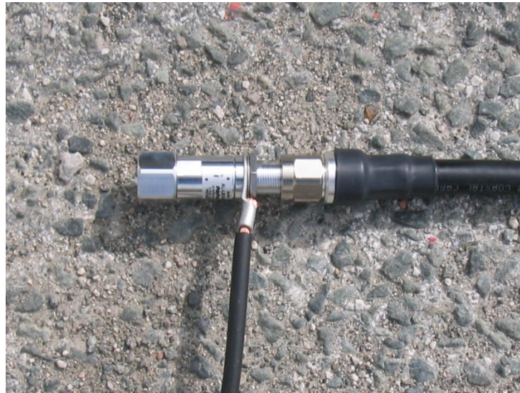
Figure 46 - PolyPhaser Surge Protector Connected to Cable with Ground Cable Attached
