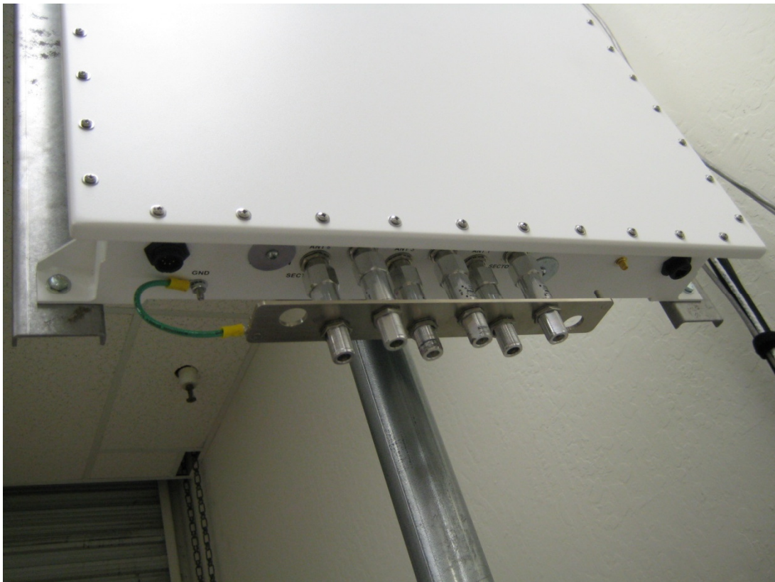
Figure 48 - Installed PureWave provides a RF lightning surge protection kit
