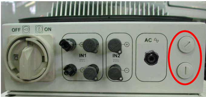
Figure 4 - Bottom of the inverter
