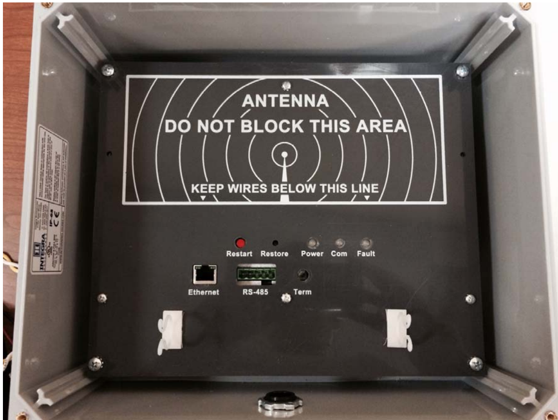
Inside SDAG Unit (with cover removed)
