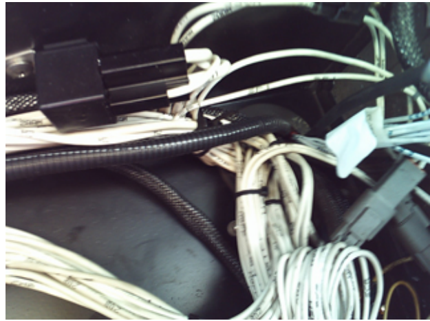
Existing Cable Hole/Gland in bottom of Controller Box which can be used for UMD Cables
