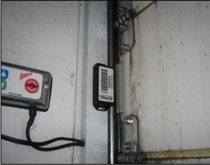
Door Tag fitted to a Roller Door Installation
