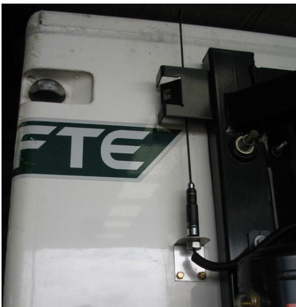
RF Antenna Location behind the Side Panel of the Fridge Unit
