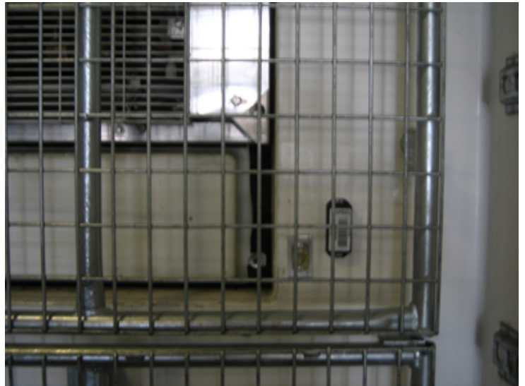
Temperature Tag located by the Return Air duct
