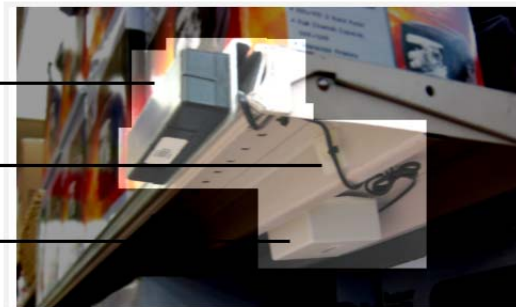
Figure 11. Installed Shelf Transmitter and Battery Unit
