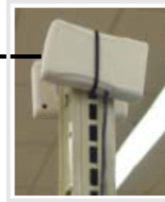
Figure 14. Installed Battery Pack/COM Unit
