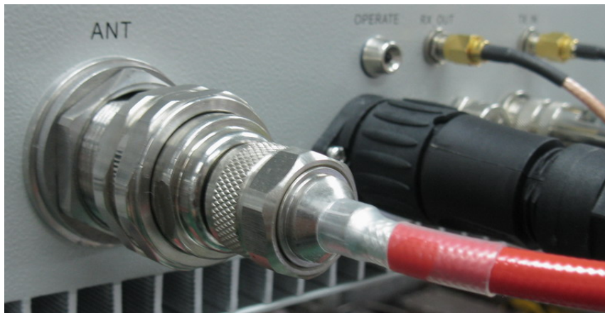
DIN(7/16) Coaxial Cable Inter-connection on Single-band RU Enclosure
