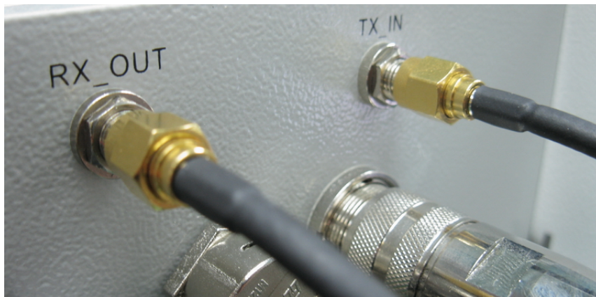
SMA Coaxial Cable Inter-connection on Single-band Enclosure
