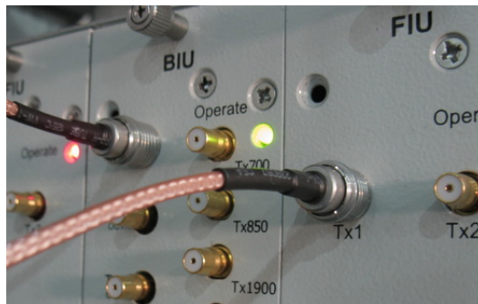
Figure 24 BTS QMA Coaxial Cable Connection
