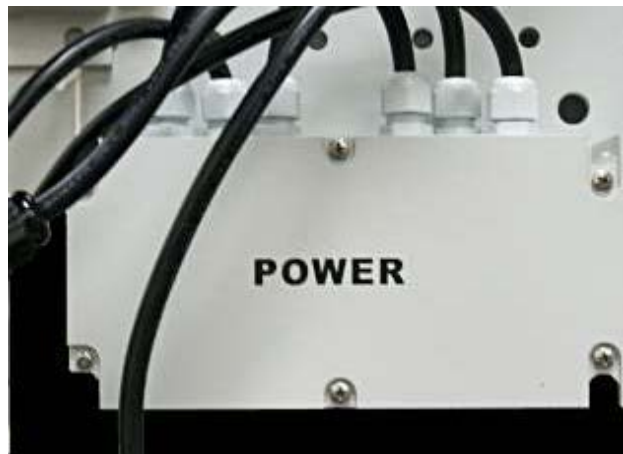
Figure 35 AC Power Junction Box
