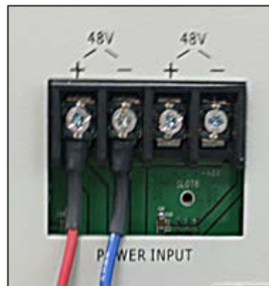
Figure 2448VDC Host Power Connection
