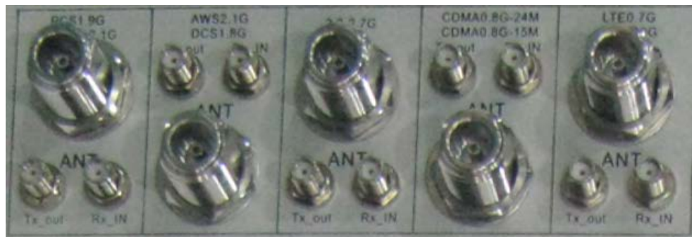
N Type Coaxial Cable Inter-connection on CM-ANT Enclosure
