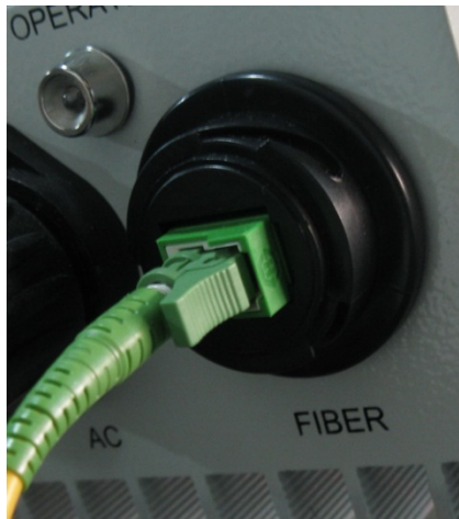
Figure 34 Fiber Optic Cable Connection to Fiber CM-BTS Enclosure
