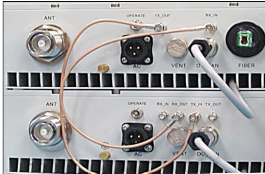
Figure 4-12. RF cable connection between Master and Slave Remote Unit
