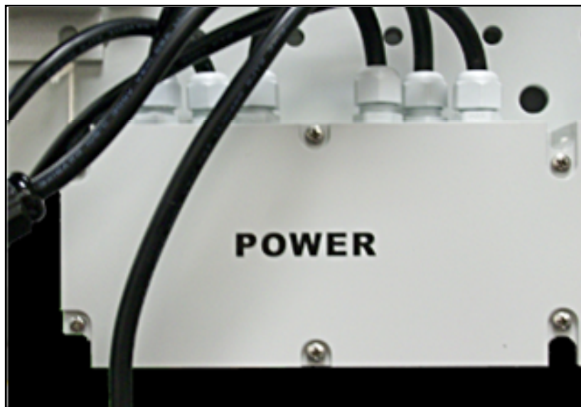
Figure 4-11. Junction Box AC Power Cable Routing
