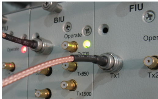
Figure 24 BTS QMA Coaxial Cable Connection
