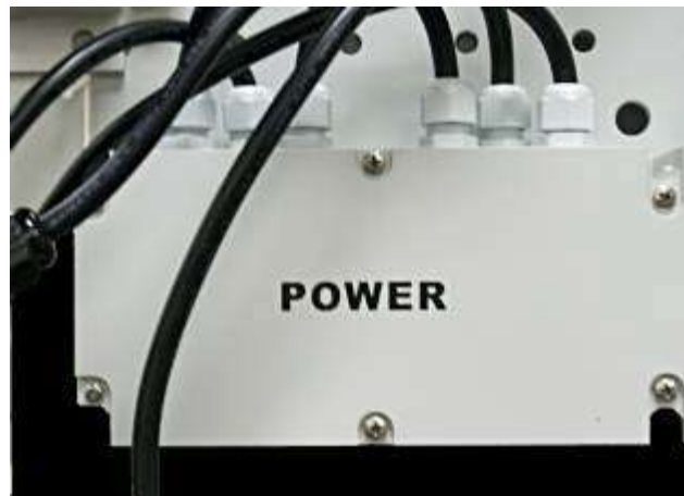
Figure 35 AC Power Junction Box
