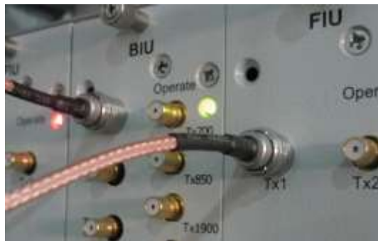
Figure 21 BTS QMA Coaxial Cable Connection
