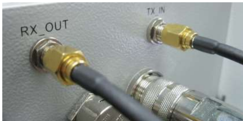
SMA Coaxial Cable Inter-connection on Single-band Enclosure
