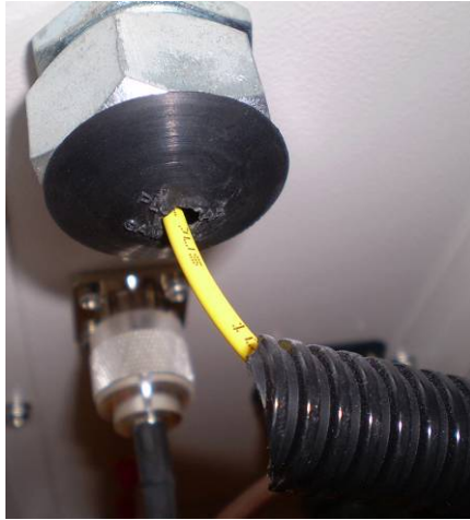
Figure 5.9 – Wrong optical port installation method
