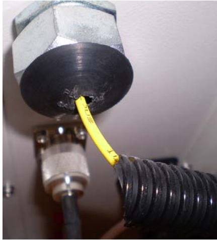
Figure 5.9 – Wrong optical port installation method
