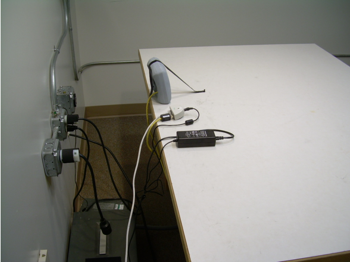
Photograph 8 – Back View Worst-Case Conducted Emissions Configuration – XAP-1010
