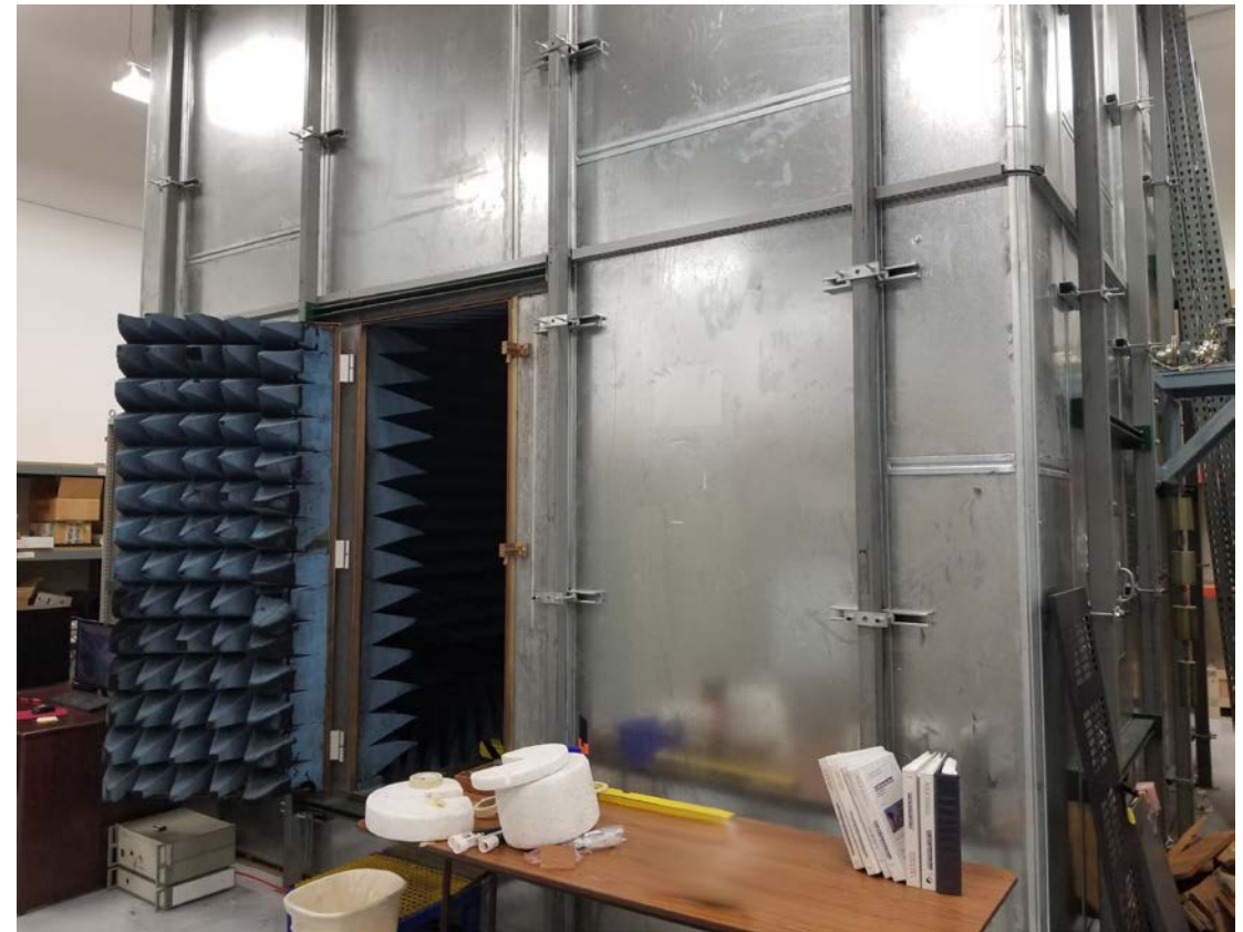
Howland anechoic chamber
