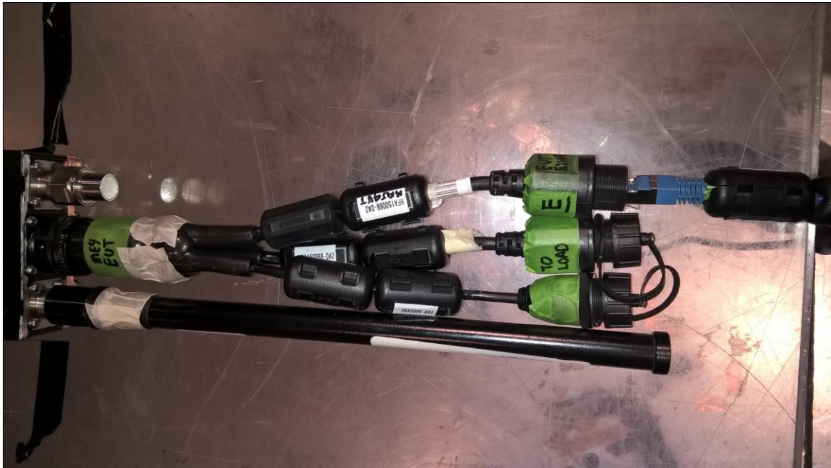
Photograph 3. Radiated Emissions Below 1 GHz, Modification to Support Equipment 3
