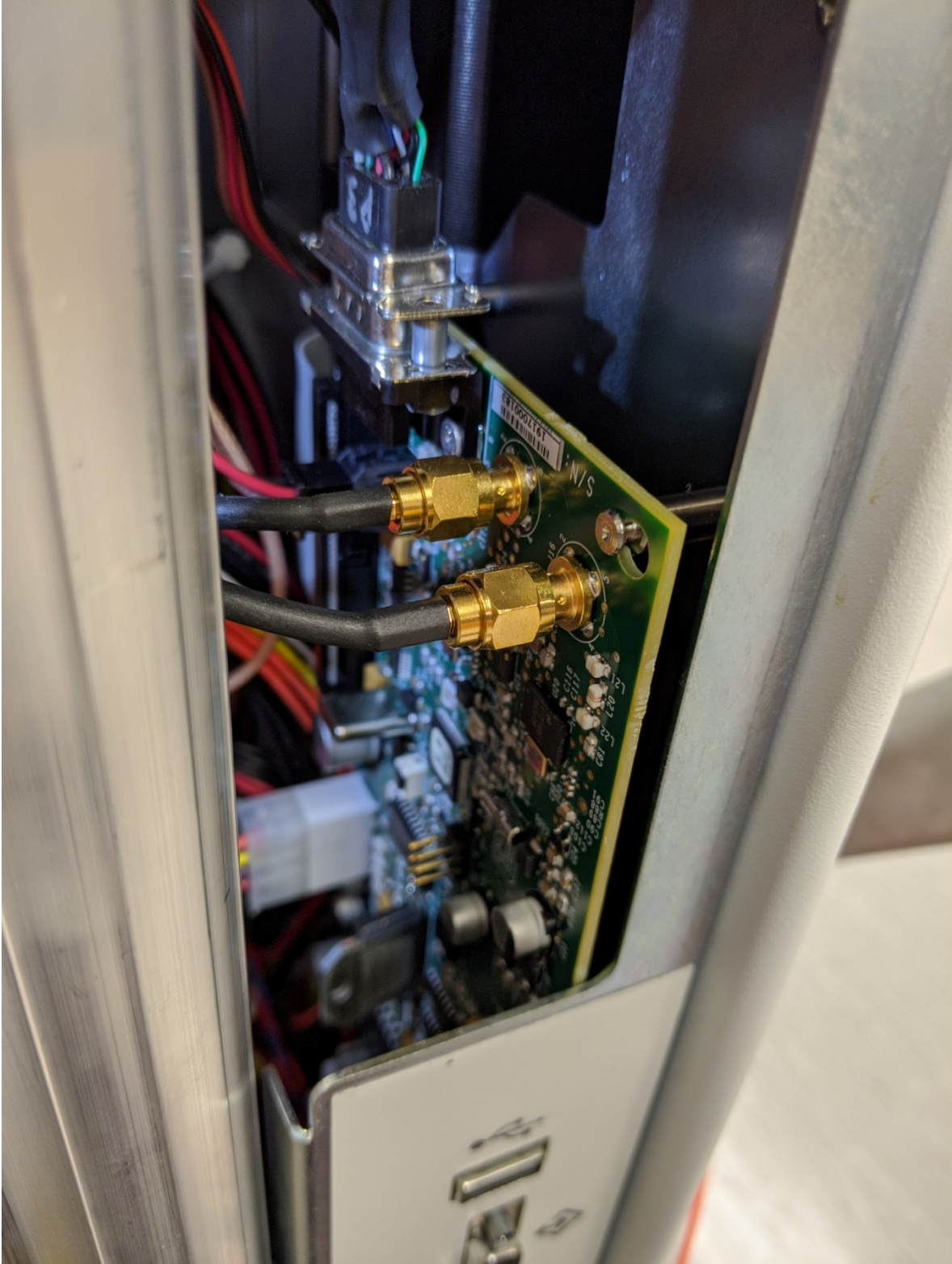
RF Module for a Bluetooth Foot Pedal control mounted in main system
