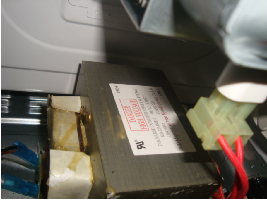
High Voltage Transformer View
