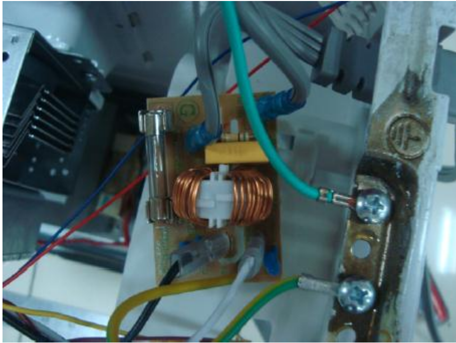
Power Filter Board Top View
