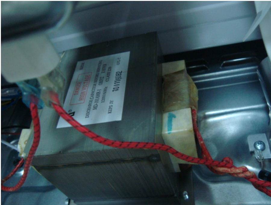
High-voltage Transformer View
