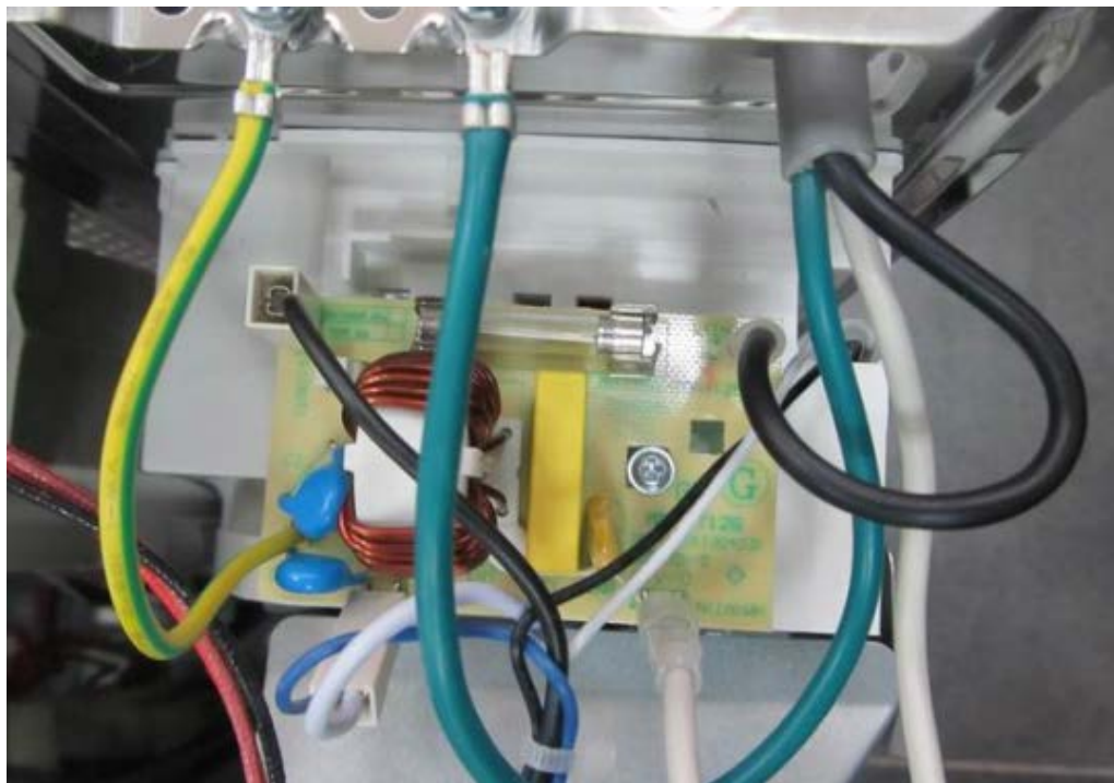
Power Filter Board Top View
