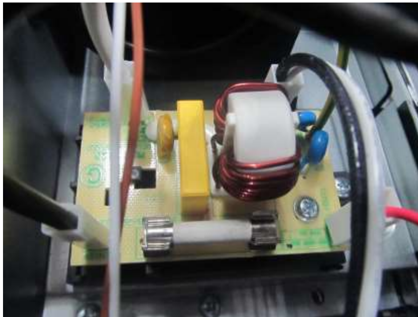
Power Filter Board -Top View
