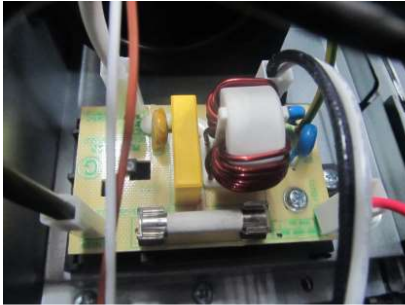
Power Filter Board -Top View
