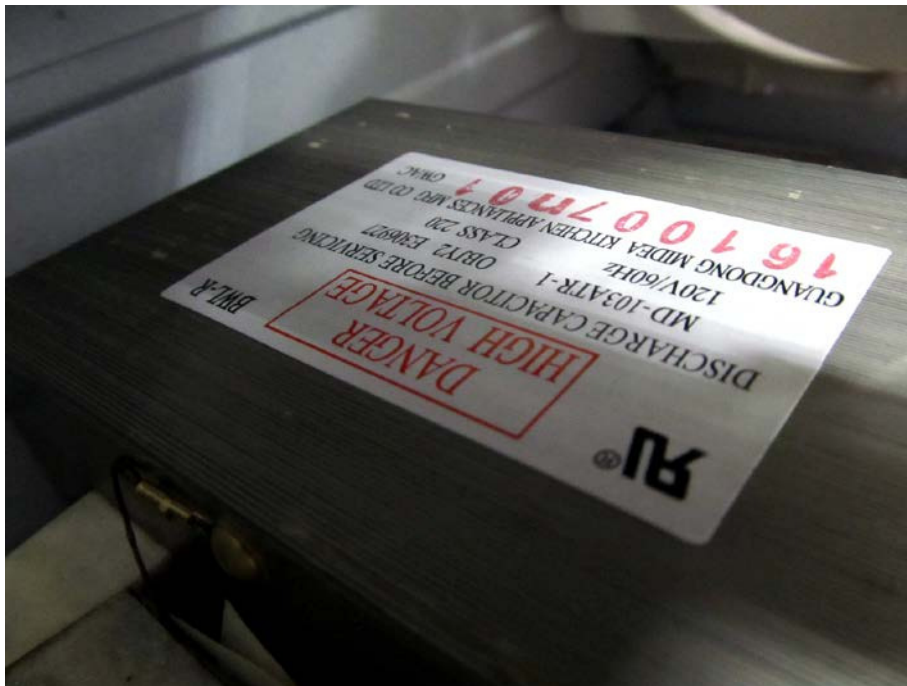
High-voltage Transformer view
