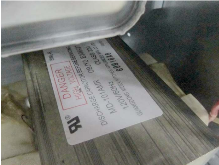
High-voltage Transformer view
