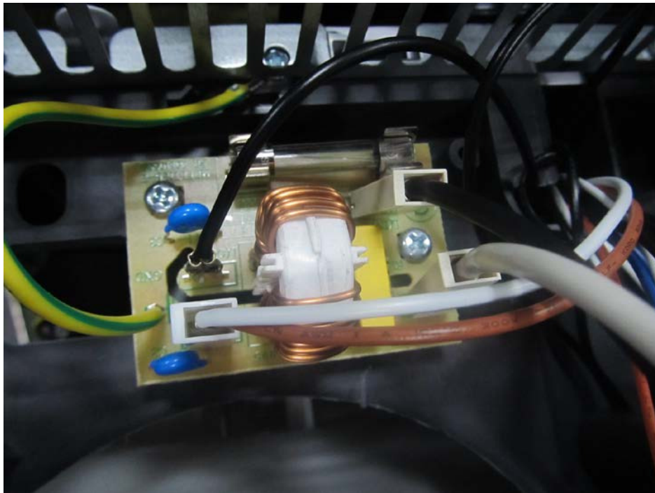
Power Filter Board- Top View
