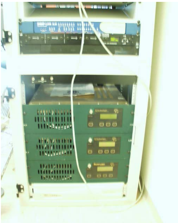
Picture 5: BSR lower rack front view (cover removed)
