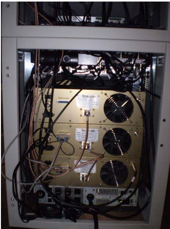
Picture 2: BSR lower rack rear view
