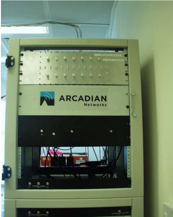
Picture 5: BSR upper rack front view (cover removed)
