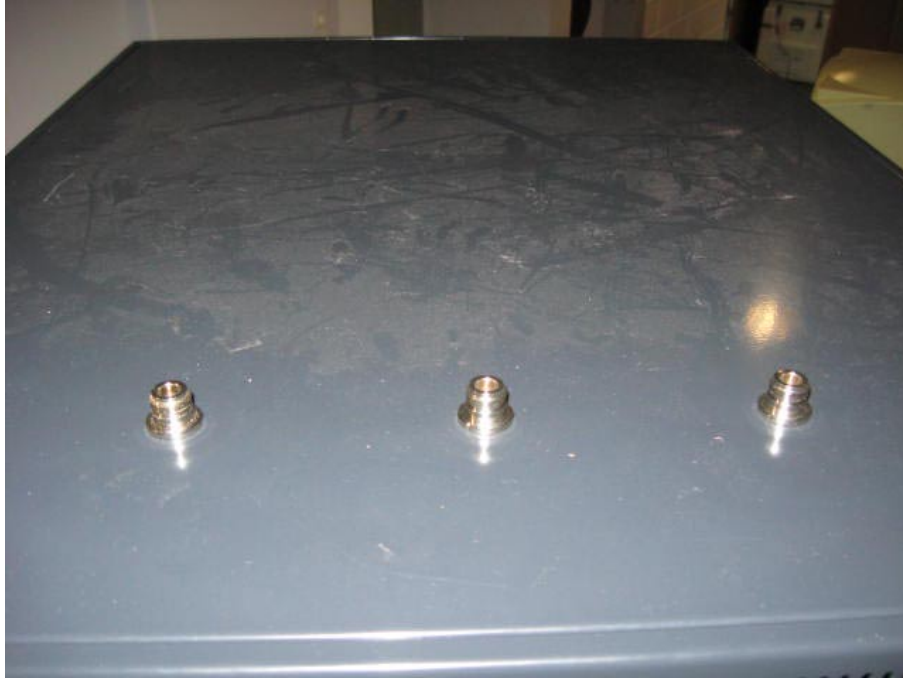
Photograph No.10 Antenna connectors external side (on top of the rack)
