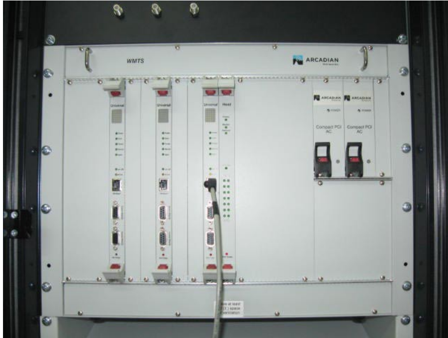
Photograph No.4 Base station ABSR-757 WMTS front view
