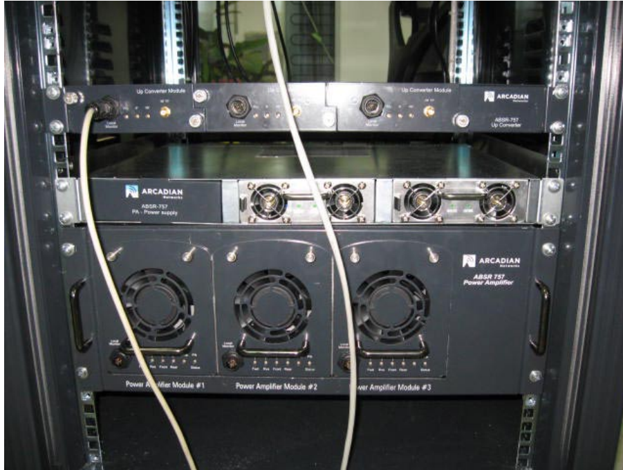
Photograph No.5 Base station ABSR-757: PA, PA Power Supply, and Upconverter front view
