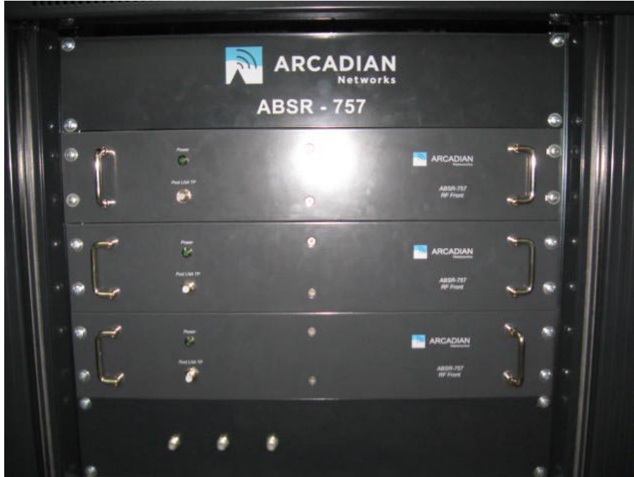
Photograph No.3 Base station ABSR-757 RF Front three sectors front side view
