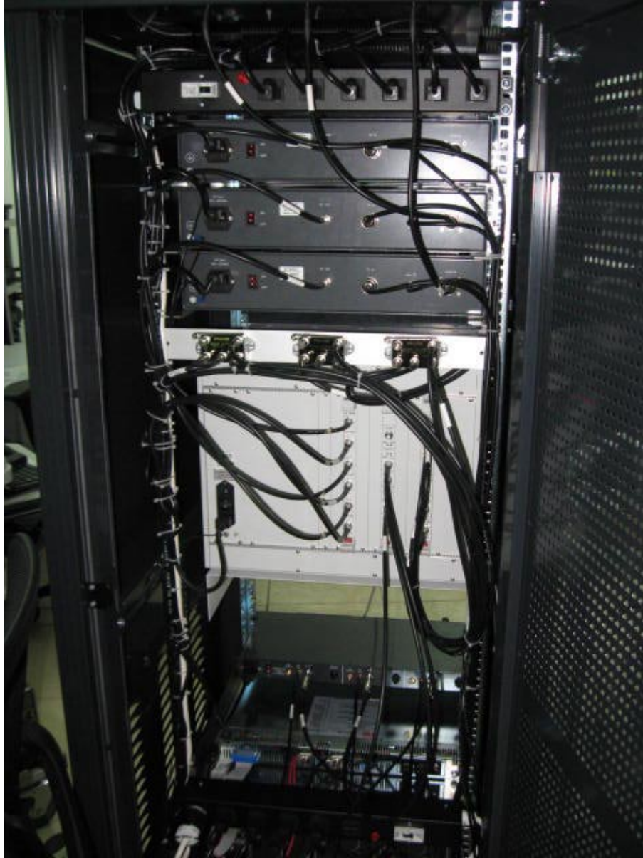
Photograph No.2 Base station ABR-757 rear side view
