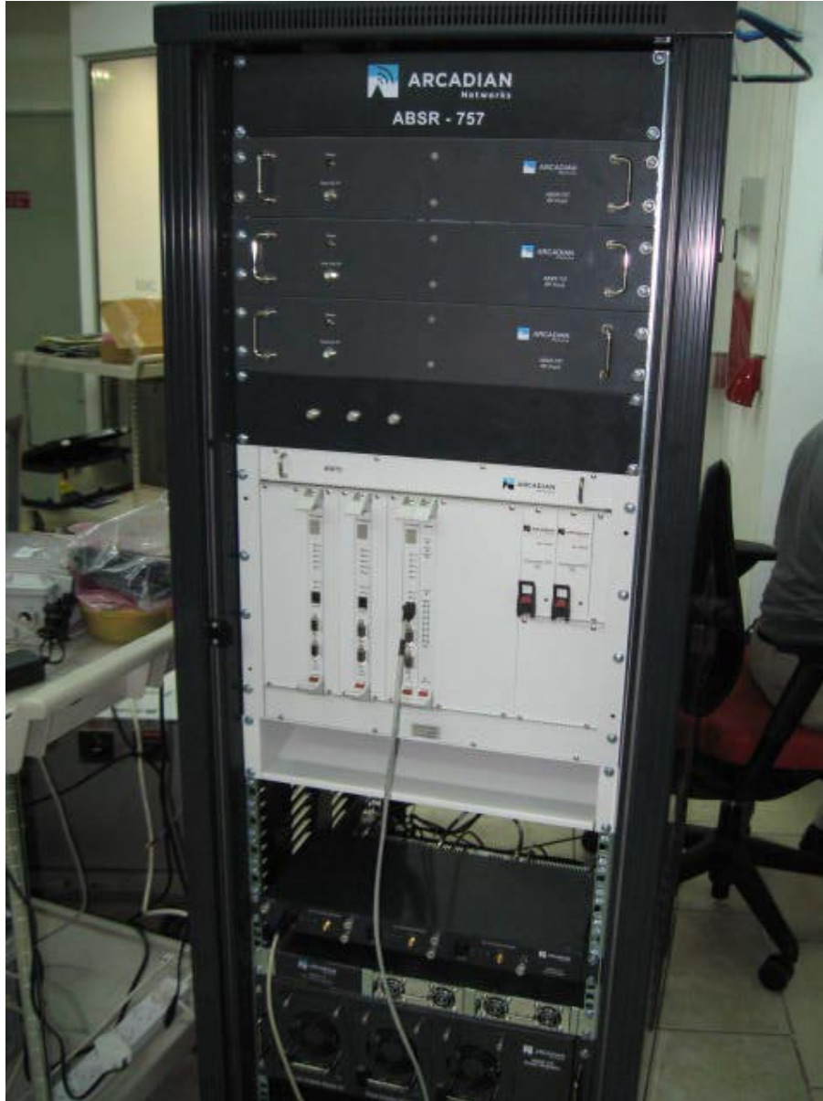
Photograph No.1 Base station ABSR-757 general view
