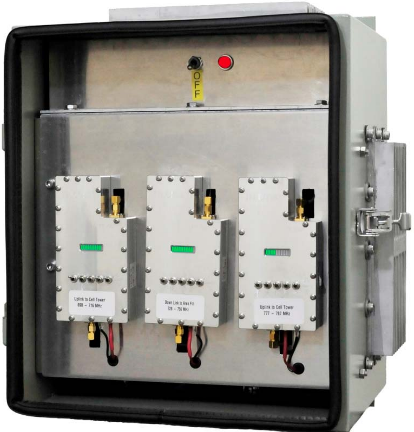
Figure E23.1 – Internal – Front Cover Removed
